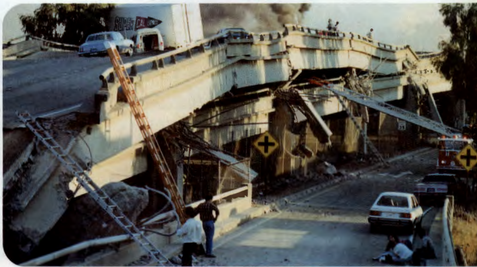
► Aftermath of the October 1989 earthquake in Oakland, California
